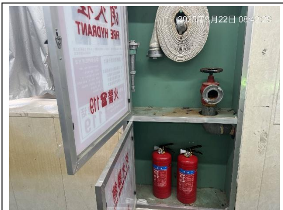
Fire hydrant and fire extinguishers
