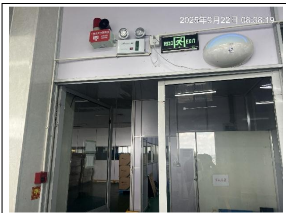
Exit sign, emergency lighting and fire alarm
