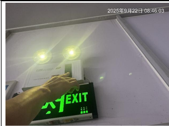
Emergency lighting test
